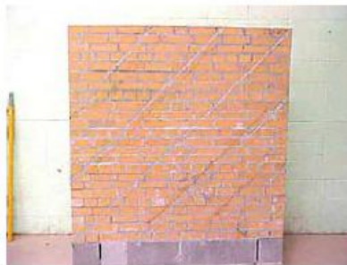
Strengthened installation with clean appearance
